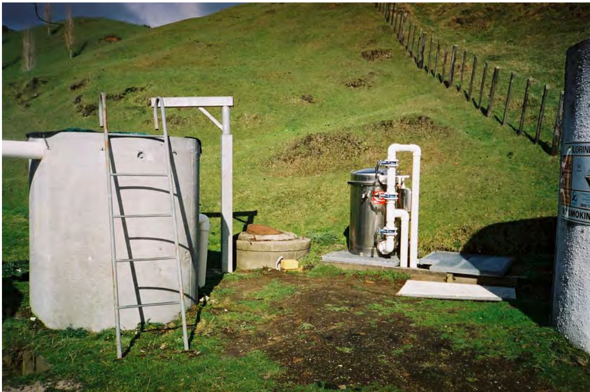
Benneydale WTP Absorption Clarifier and DE filter 2008
