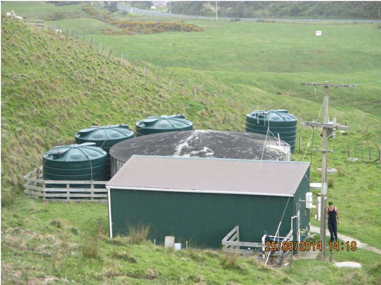
5Mokau WTP and Storage Reservoirs
