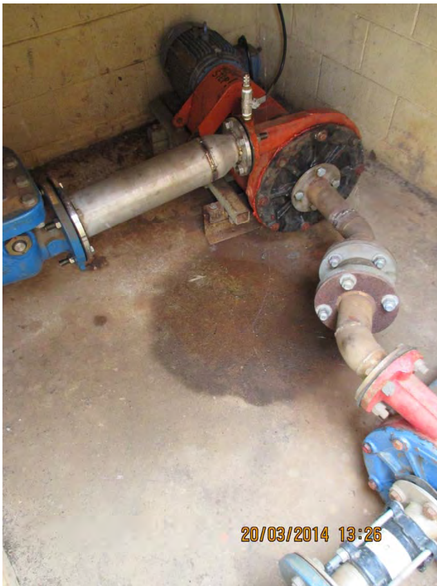
4Awakino Hill Pump Station
